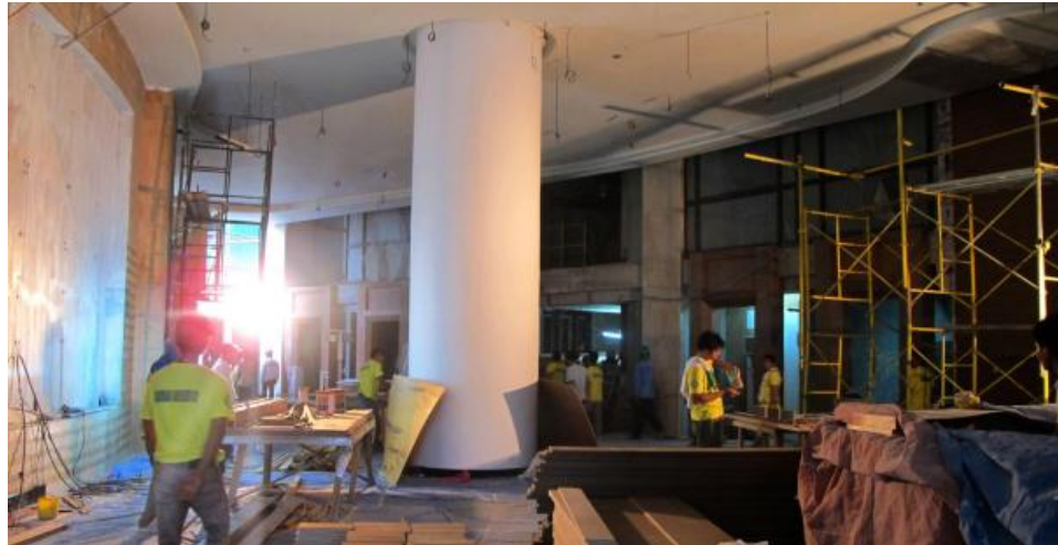
The Knightsbridge lobby takes shape as it continues fitting-out activities in November.
