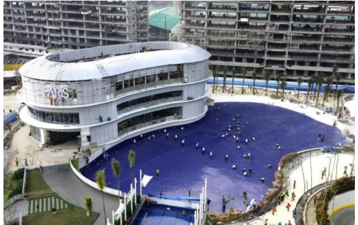
Tiling works have finished at the Azure beach. Beach sand laying is in-progress.
