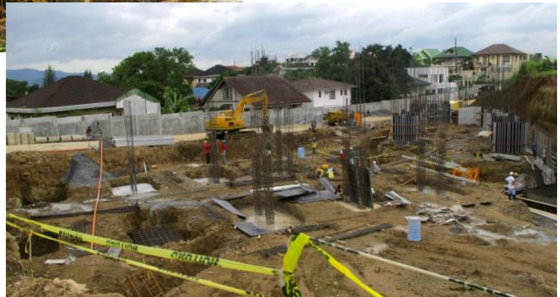
Substructure works and concrete pouring for column footings at the site of the third tower, Osmeña East
