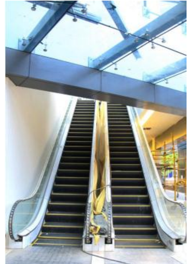
The building's escalators, such as this one along the Kalayaan Avenue main entrance, are fully installed.
