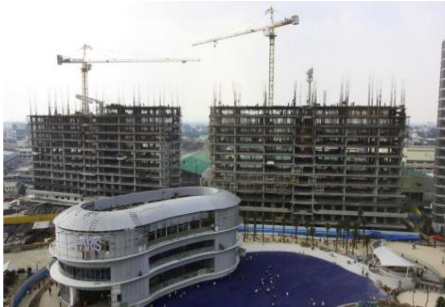
Positano (right) and Miami (left) are each on the 14 th level of structural works
