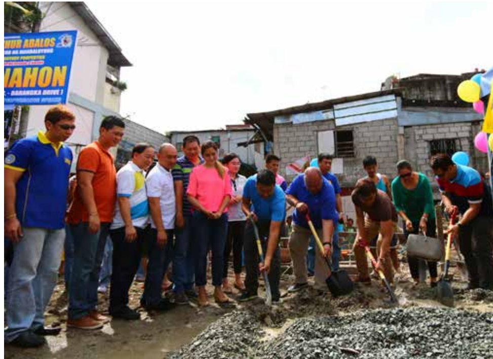
The official commencement of the GK-Century Properties Village construction in Hinahon St., Barangay Barangka Drive, Mandaluyong City were led by (foreground from left) Gawad Kalinga Executive Director Jose Luis Oquinena, Century Properties Vice President for External Affairs Resty Ingal, Mandaluyong City Mayor Benhur Abalos and Mrs. Carmelita Aguilar Abalos, joined by city council and barangay officials of Mandaluyong, and officers of Gawad Kalinga and Century Properties.
