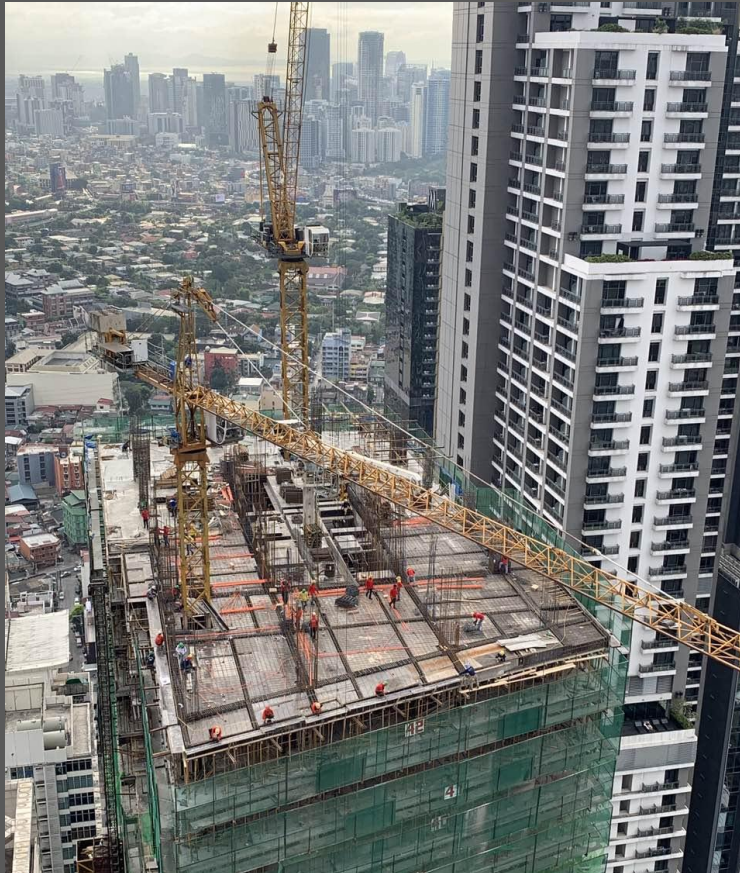
Formworks and rebar works ongoing at the 43 rd floor of Century Spire
